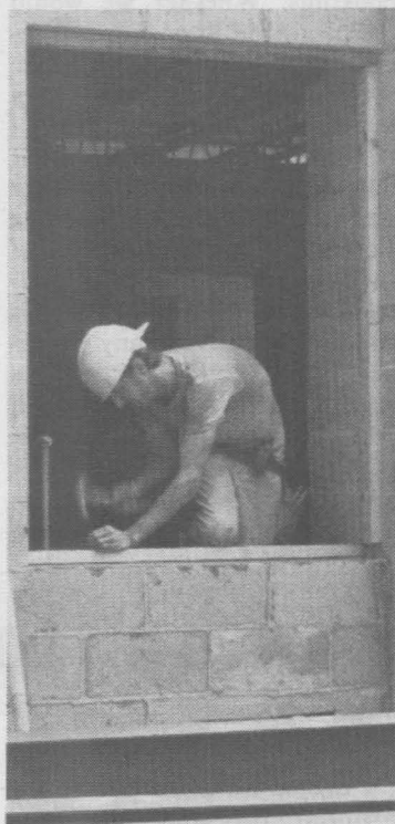
INSIDE LOOKING OUT —A worker frames a window in one of the new women's residences. [Photo by Nathan Faulkner]
